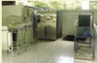
Autoclave do Aeroporto de Manaus The Autoclave of Manaus Airport
